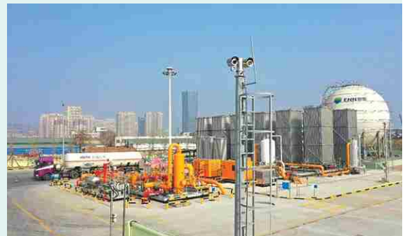
ENN Qingdao Tuanjie Road Plant applies LNG Unloading Safety Vehicle Supervision Solution
